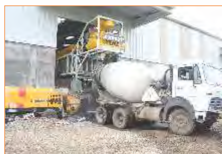
Pump & TM Application
