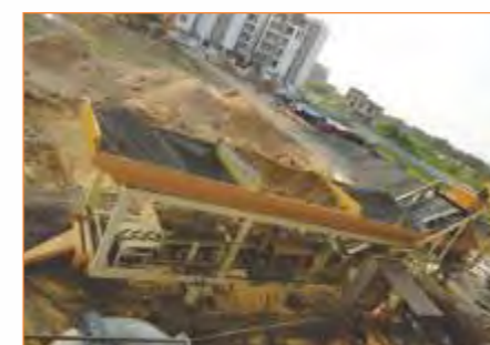
In Line Storage Bins
